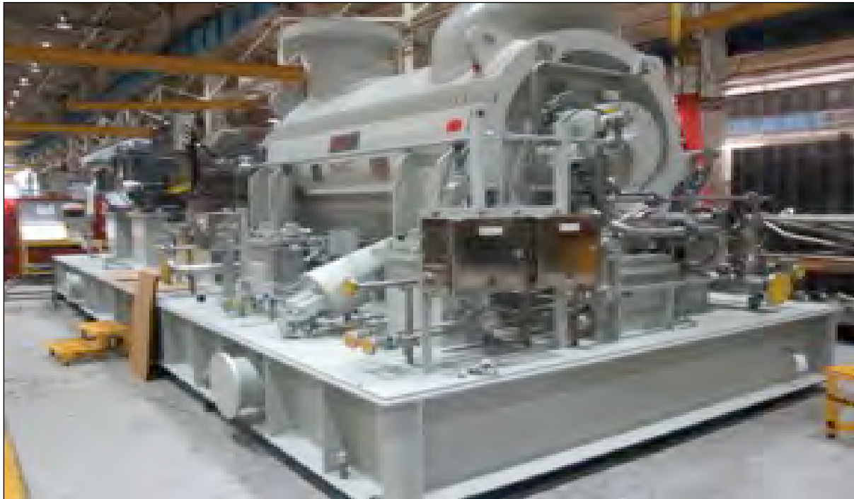
Figure 13.15 Main air compressor (Elliott Group model 46M6I)
